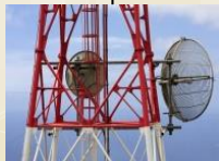
Base Station Mobile Phones
